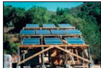
Photo Courtesy of Solar Electric, Inc.
